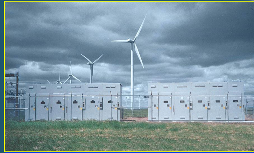
Interconnection with 25 kV Metal-Enclosed Switchgear
