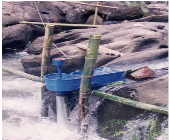
Fig. 7. Pico hydro unit in Ecuador
