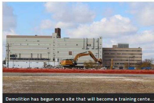
Demolition has begun on a site that will become a training center...
