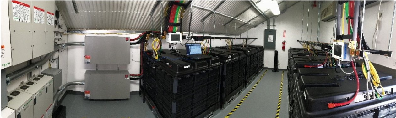
Energy storage system at IIT nanogrid
